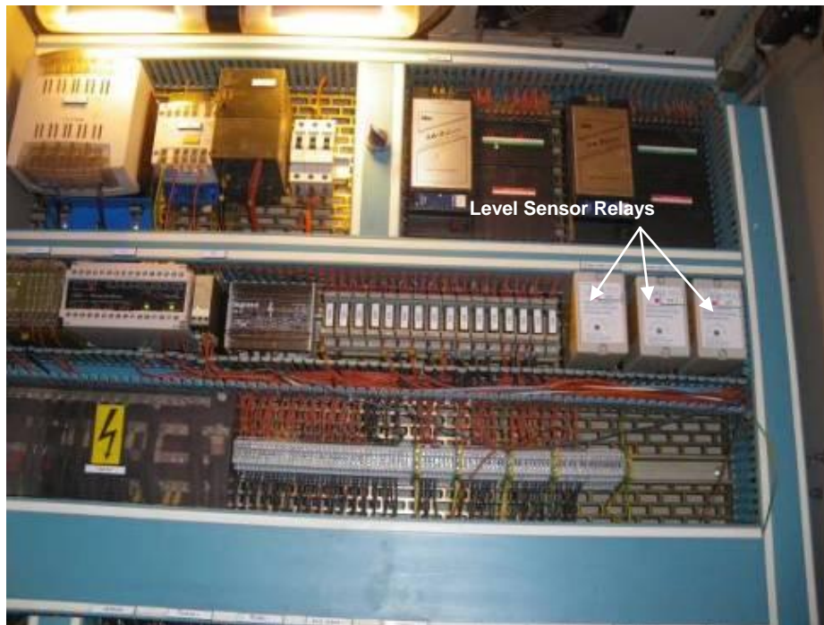
Level Sensor Relays in Electrical Control Panel
