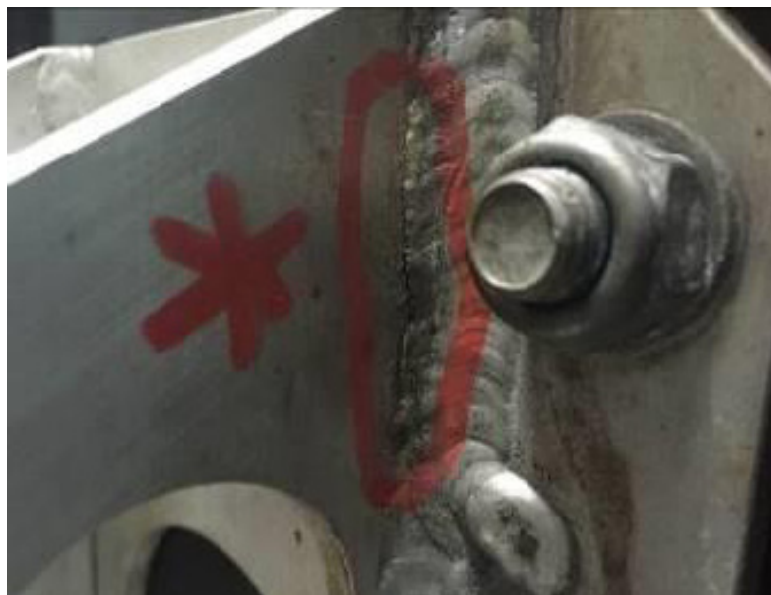
▲ Cracking on a vertical weld – found by DPI
